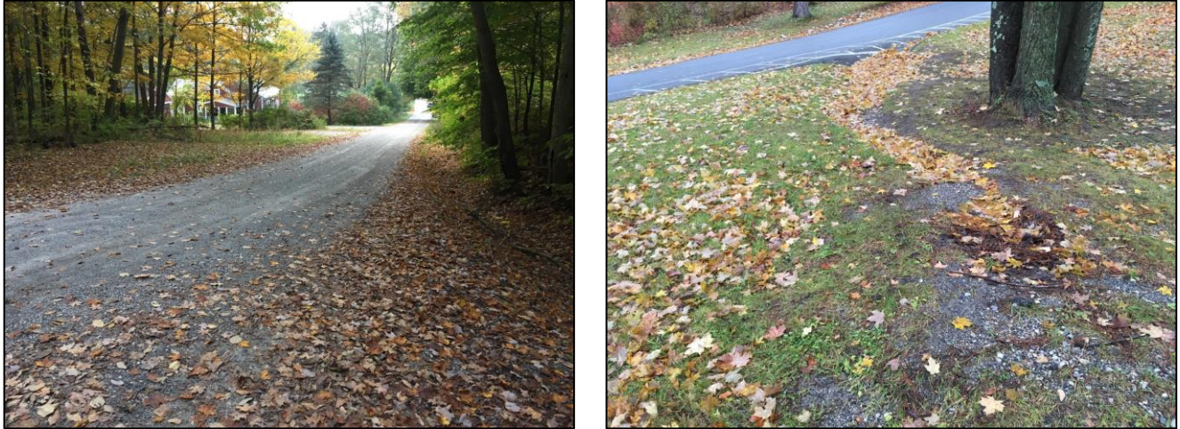
Figure 5.1: An unstable drainage ditch on the southern section of Tory Lane was tied for the lowest individual score (RD-15). An eroded flow path to a catch basin receiving runoff from impervious areas at Arlington Memorial High School (SW-12) was tied for the highest problem area score.
