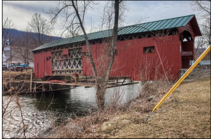
Figure 3.1: Post-Irene repairs in progress at the West Arlington covered bridge. Photo by Harold Stiver.
