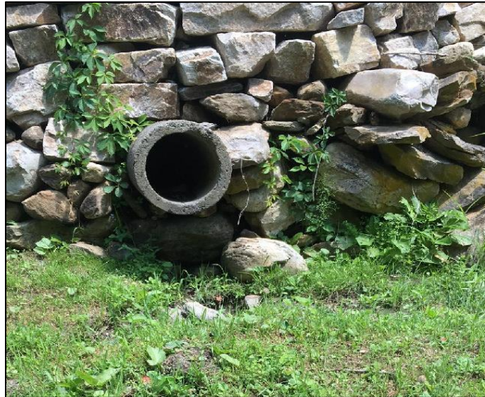
Figure 4.1: An outfall that “Partially Meets” the REI standards due to rill erosion at the outlet.
